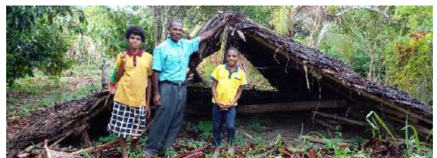
13 years of weather took its toll on the original lamb shelter.
